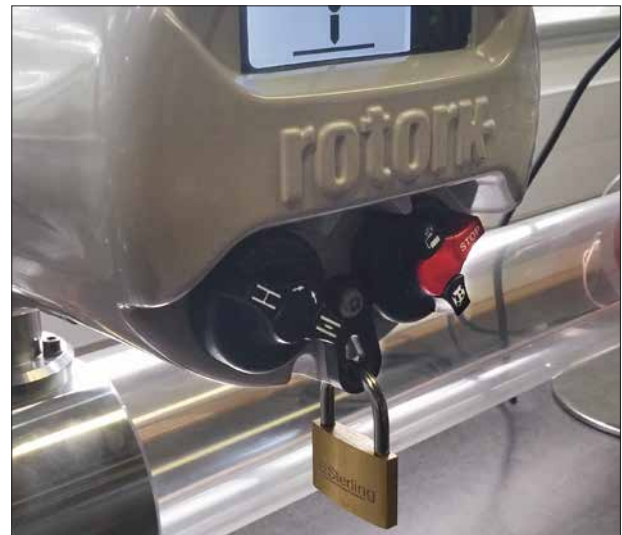
Fig 7.2. IQ3 control selector padlocked in "Remote"
