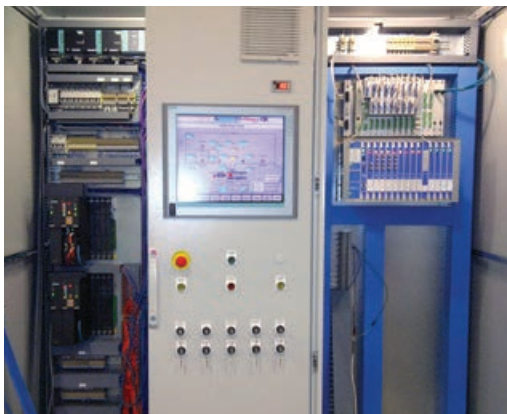
SIL-2 PLCs with interactive touch-screen color HMI and BN monitoring systems inside a control room
