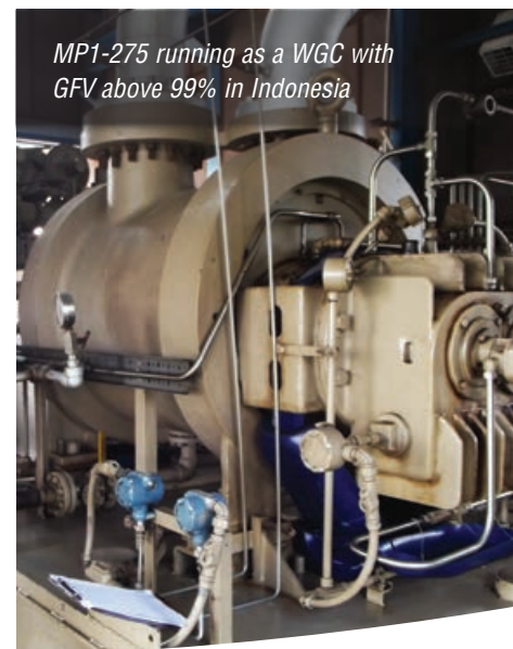
Engine-driven MP1-430 installed off the coast of Turkmenistan in the Caspian Sea undergoing a string test
